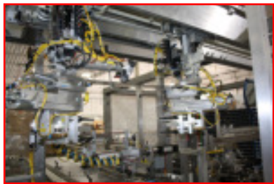
Innovative Infeed System for this application denested support trays, picked and placed booklets, and handled filters and then end load all three items
