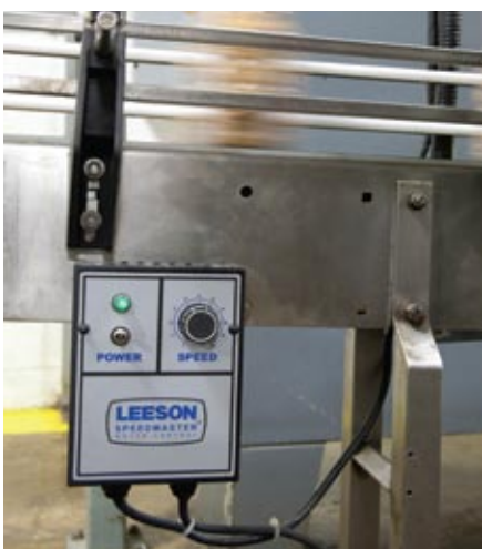
A Leeson Speedmaster controller ensures that the product on the conveyor system is always moving along the bottling line at operating optimal speeds.
