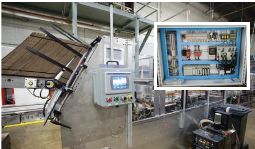
Utilizing Rockwell Automation's Allen-Bradley controls (inset), an AFA Nordale tray-loader is a key Johnvince Foods capital investment that enabled the nuts processor to reduce its secondary packaging waste.
